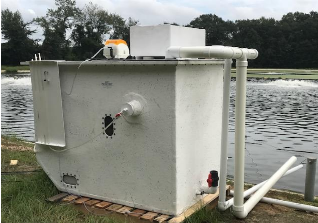
Figure 9. RCPG ® 10 was designed for on-site sizing evaluations. This unit is positioned next to a lagoon, linear air pump powers the backwash, unseen rotary vane air blower drives the airlift. Splitter box and PSE sludge discharge lines visible on top and pitot tubes on side for head loss evaluation on recirculation loops.
