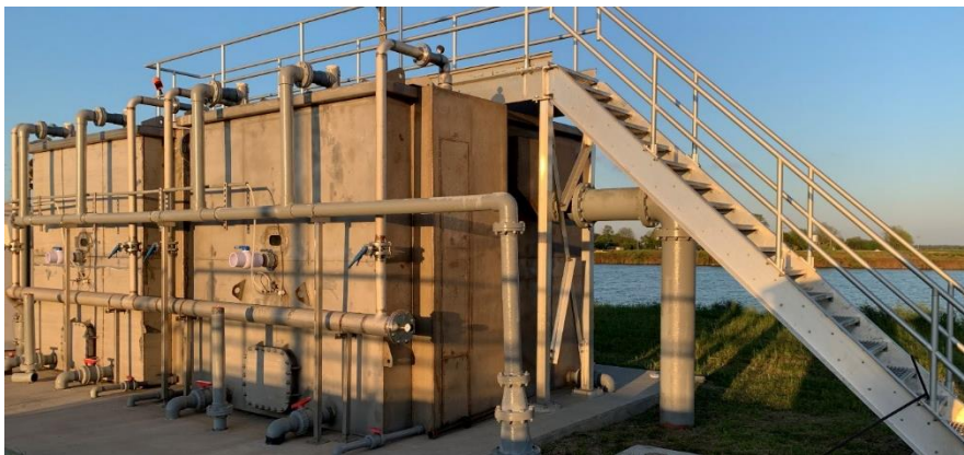
Figure 4. Two RCPG ® 250s installed in series to control ammonia discharges on a domestic lagoon system in northern Mississippi.
