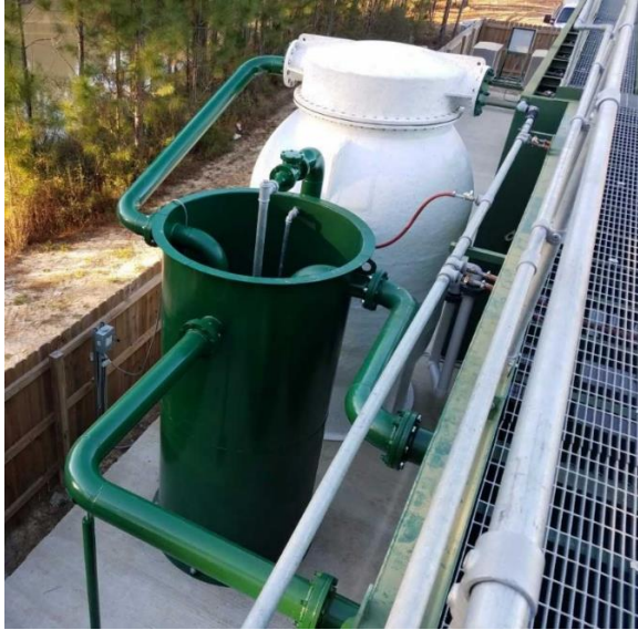
Figure 3. The early recirculating models used a separate tank as a reservoir. Flow was driven by a pump with aeration by spray head, Venturi, or packed column. This unit is attached to a package treatment plant servicing a subdivision and assures new stringent ammonia standards can be met.
