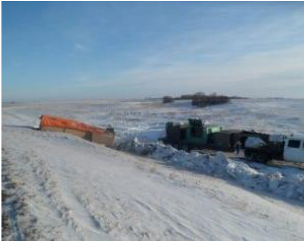
4-ft x6-ft and 4-ft x 8-ft panels, made of plywood and rigid insulation were used to build walls around the culvert ends, and the walls were covered with insulated tarps to create large hoardings.
