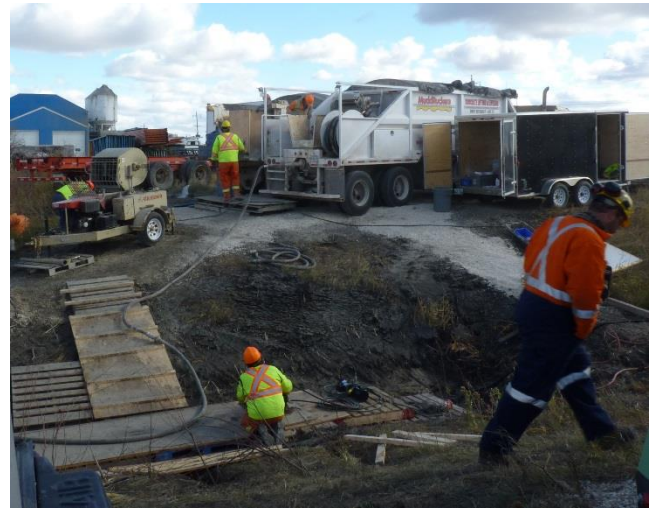
Site prep and staging included dewatering and a network of pallets to provide secure footing on the muddy terrain
