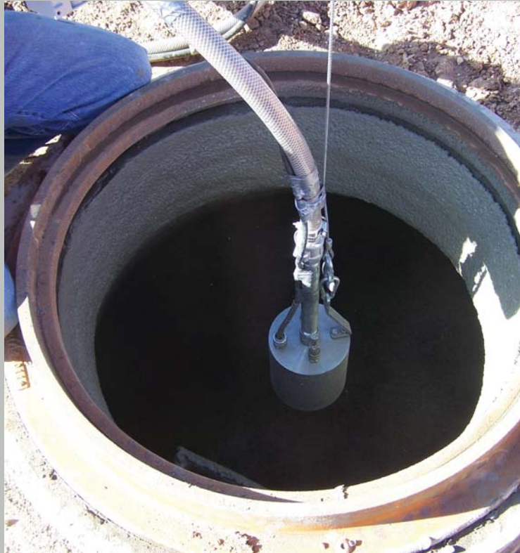
The SpinCaster makes 20 to 30 passes through the center of the manhole's axis.
