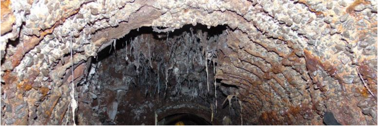
Top half of interceptor, completely rotted out and held in place by root masses
