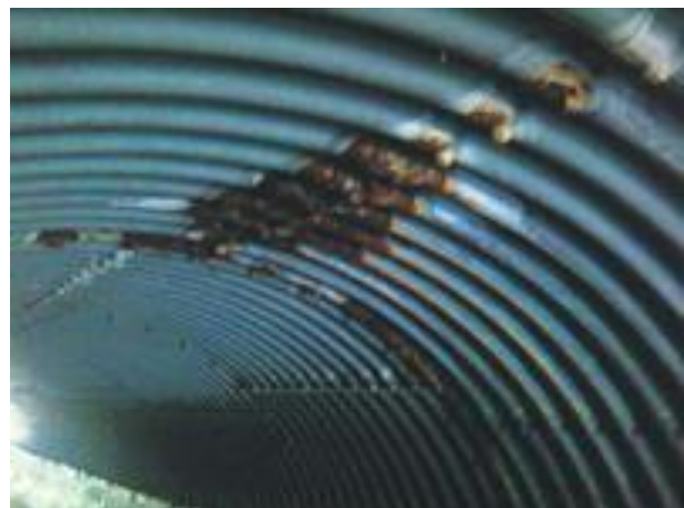
Culverts made of bolted corrugated metal plates sometimes fail at seams and boltholes.
