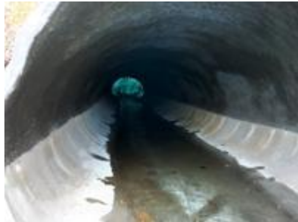
A completely rehabilitated arched metal culvert; the upper arch was spraycasted with cementitious grout.
