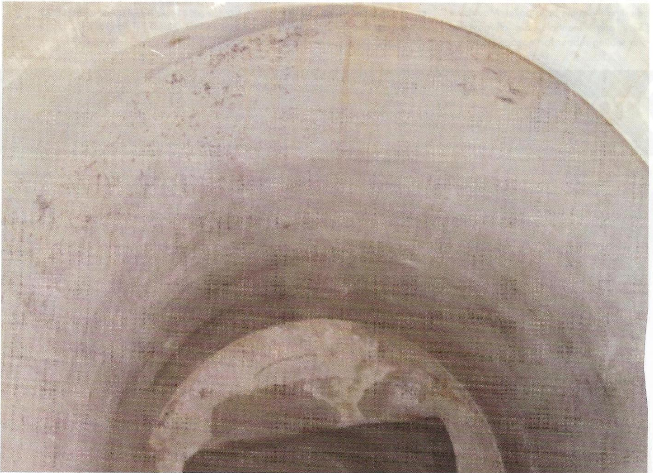
Nine-Year Test for Corrosion Protection Proves Benefit of ConmicShield® Additive in Concrete
