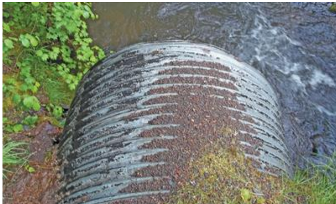
The 526-ft overflow culvert runs parallel to the west side of the highway and is made of 72-in. corrugated metal pipe.
