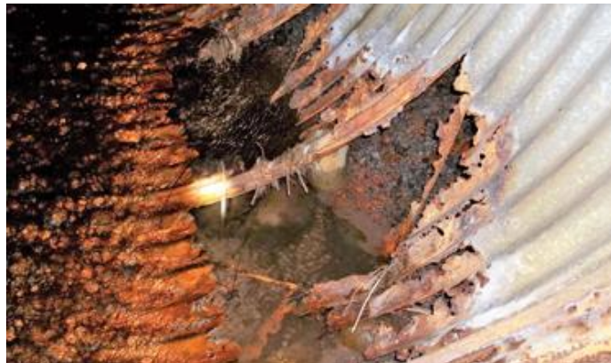
Before rehabilitation, the corrugated metal pipe showed signs of physical damage due in part to storms and debris pushed through by high-velocity flows.
