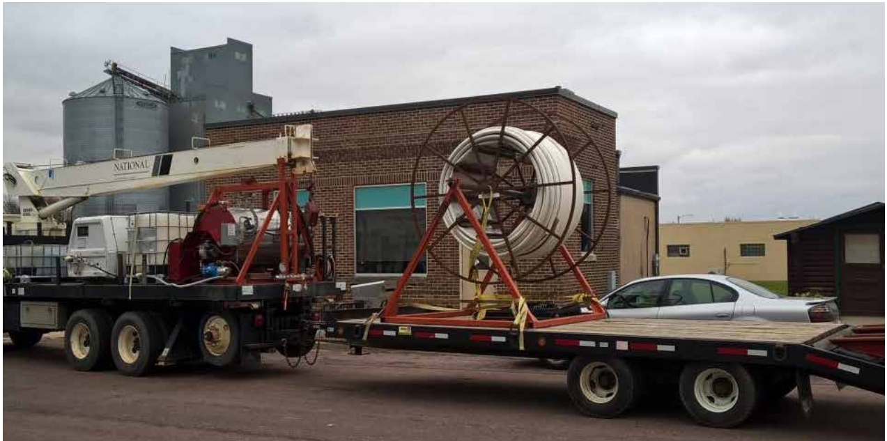
Boiler truck/Air compressor and Reel on A-Frame on Flatbed trailer at A-side
