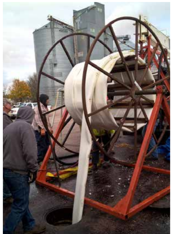
Liner de-reeled and pulled through on A-side, showing remaining liner on reel
