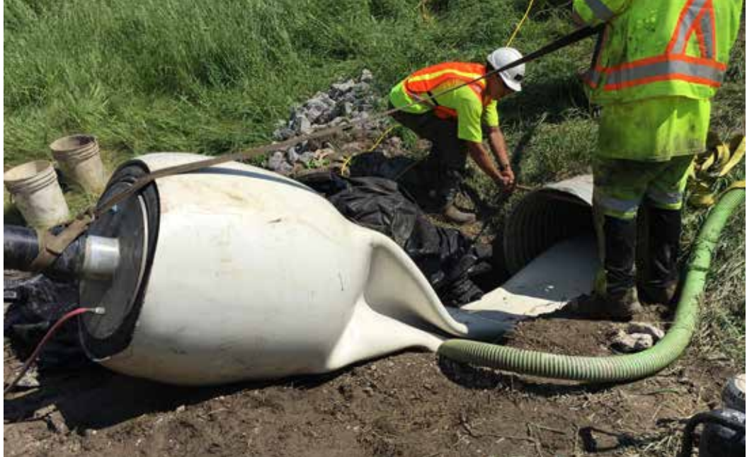
Reel is heated with steam to make the PVC flexible to slip through the inside of the culvert
