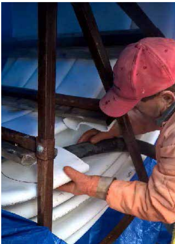
Positioning the steam hose at liner inner end to prepare for inflatable plug insertion
