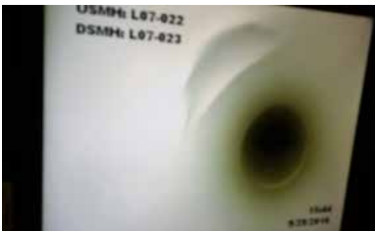
CCTV snapshot of relined host pipe with "dimple" showing at 4" service lateral
