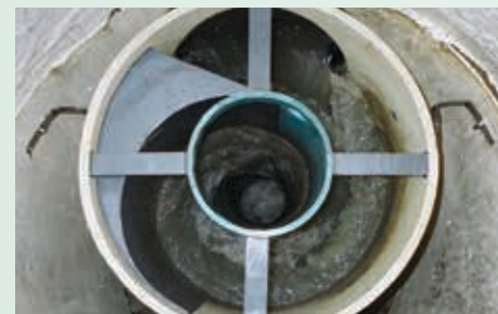
Vortex Flow Insert reducing H 2 S concentration levels, Camden County, New Jersey.
