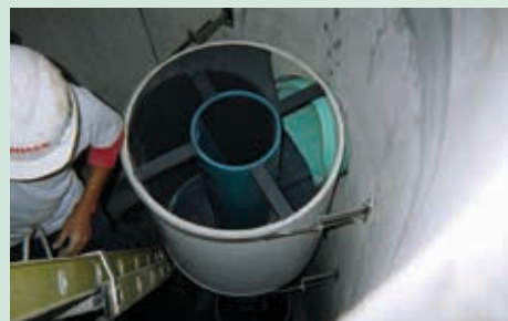
Stainless steel straps and epoxy painted walls for additional layer of corrosion protection, Charlotte, NC.
