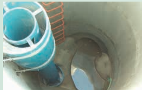
Second effluent line at bottom, benching from the EDP to direct flow, Sarnia, Ontario.
